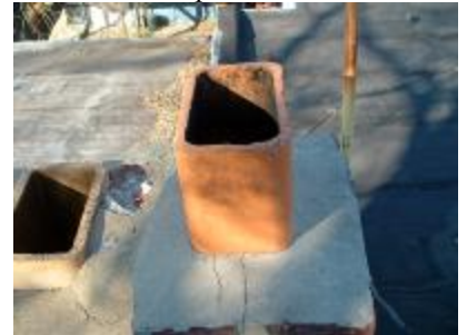
Seal cracks in the cement wash... Install a rain cap and vermin screen...
