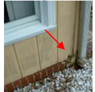
Rot at siding...
