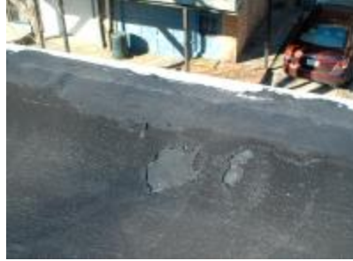
Main roof...damaged areas...
