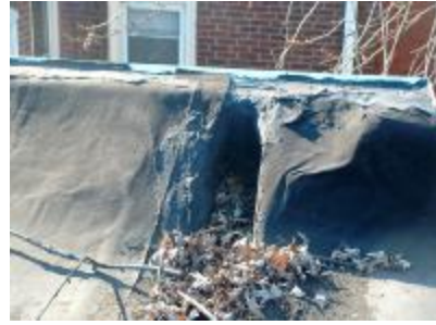
Congested roof drain...
