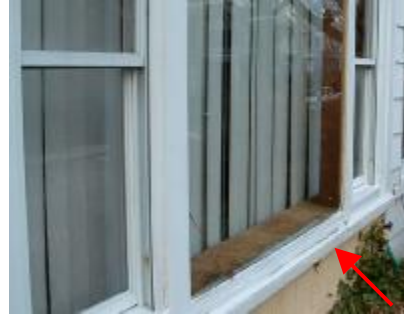
Rotted...frames, trim and sills...
