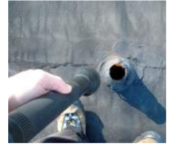
Pipe...open into the attic...
