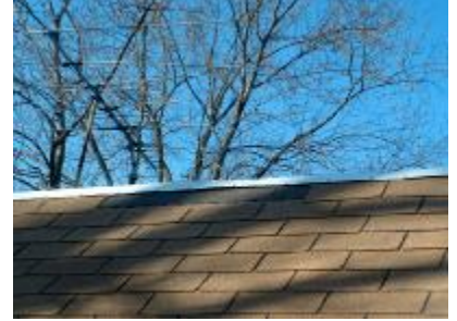
Shingles are missing...
