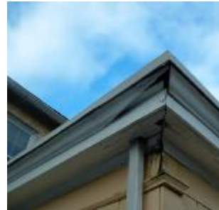
Rot at eaves...
